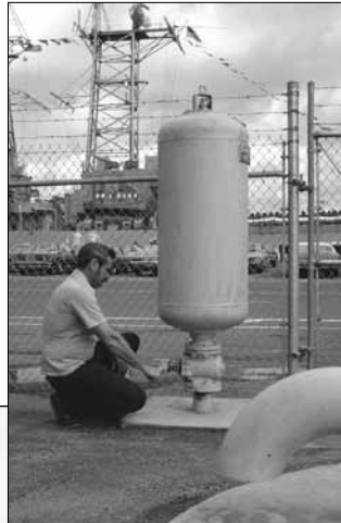
Refineries — Shock from pump starting and stopping
