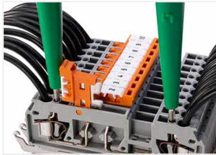
Testing with voltage tester.
