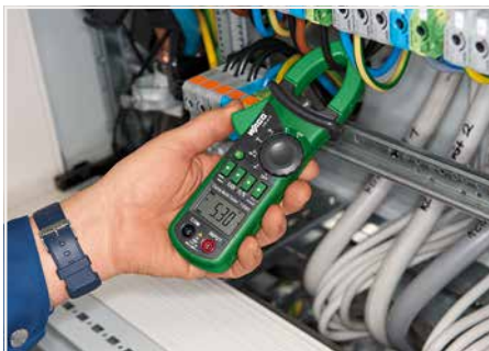
Voltage testing in control cabinet
