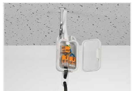
Pendant light connection in suspended ceilings
