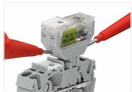
Testing via 2-pole test plugs.
