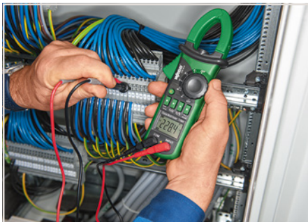
Current measurement in a control cabinet
